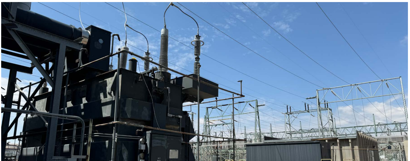
Transmission line infrastructure at Naughton Power Plant.
